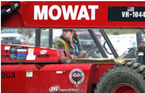
LUI KIT WONG/THE NEWS TRIBUNE Angie Rennaker of Graham, 20, operates a 10-ton, high-reach forklift while moving construction materials for the light-rail project at Sea-Tac Airport.
